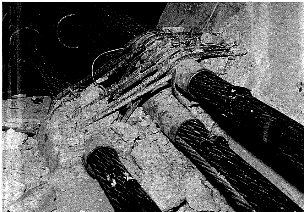
Figure 6.16 Block A: Immediately After Failure
