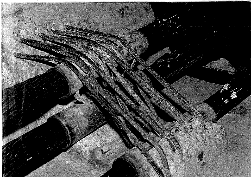
Figure 6.17 Block A Failure: Details
