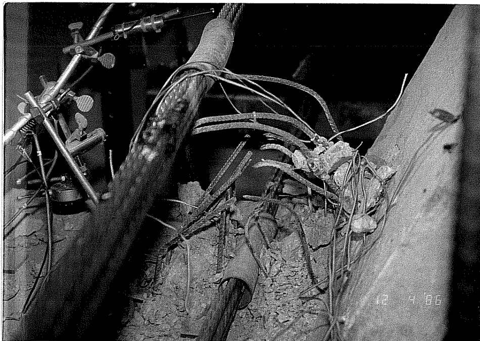
Figure 6.11 Block B: Immediately After Failure
